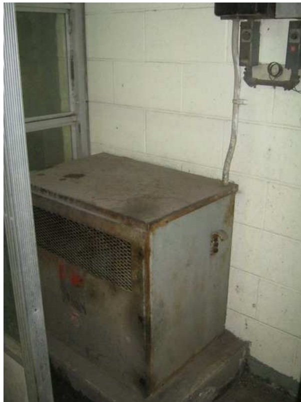
D501004b 33kVA transformer in bus shelter in wash bay
