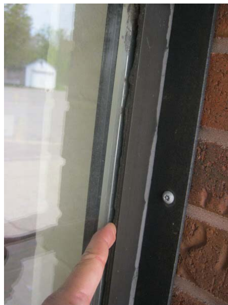
B2020c Fixed window missing exterior glazing tape
