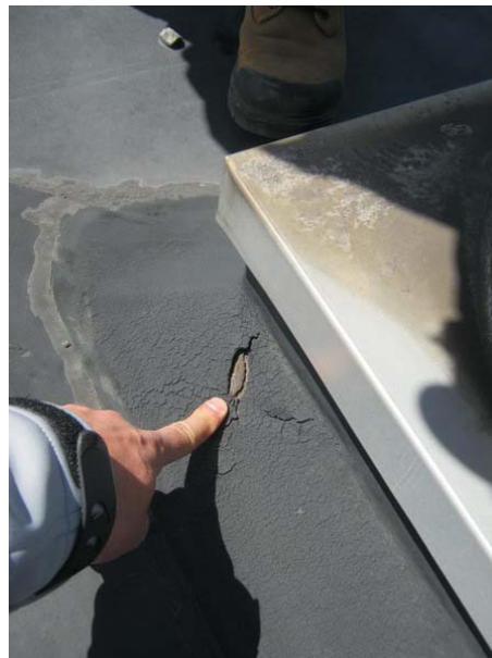
B3010b Visible penetration through roof membrane
