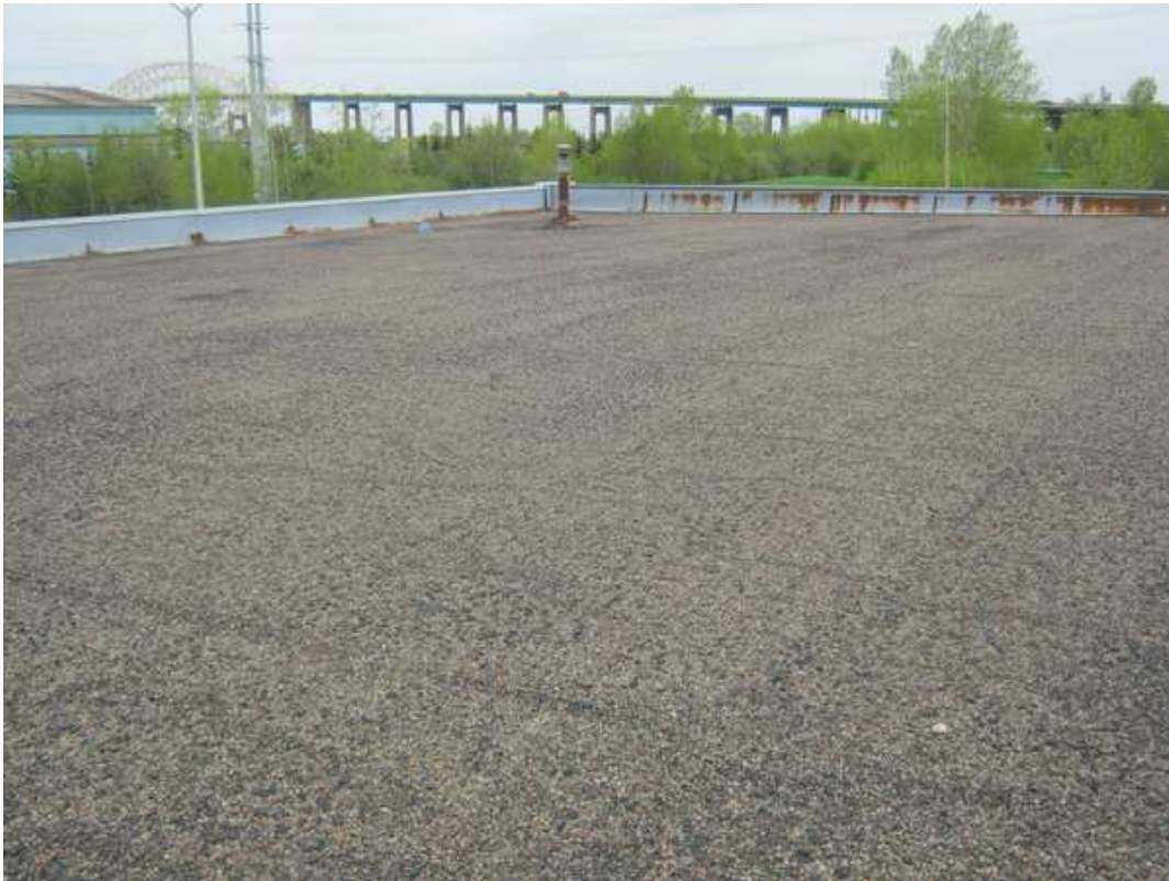
B3010a Overview of typical ridging and exposed felts at garage roof
