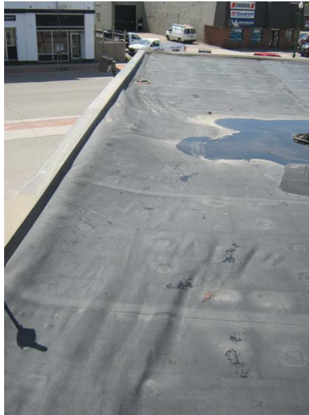
B3010c Tenting and wrinkling of roof membrane at edges
