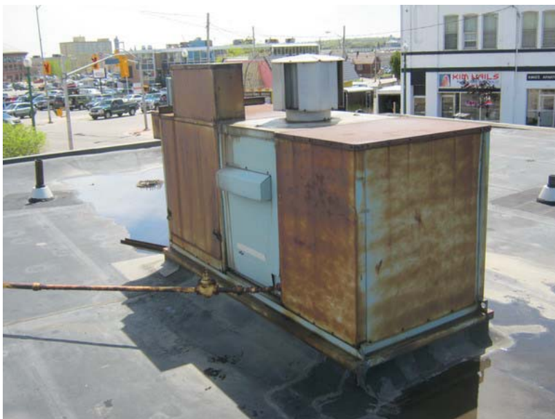
D3050 Original rooftop heating unit
