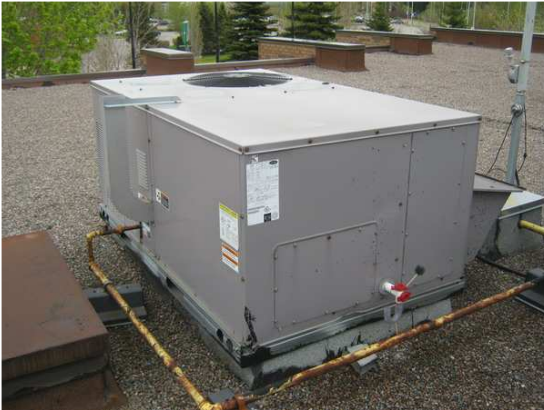
D304008-1 Typical Newer Carrier Rooftop unit at Office
