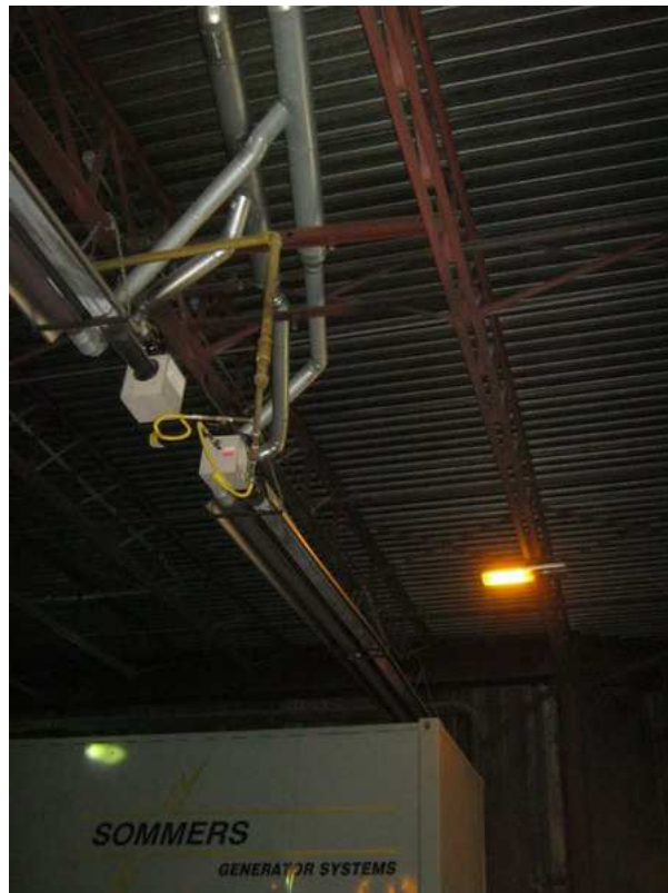
D302004 Typical Newer Radiant Heaters at Storage Garage
