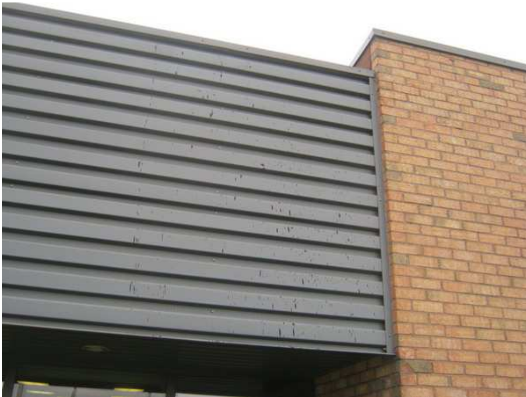
B2010b Corrugated Metal Cladding, Showing Asphalt Staining
