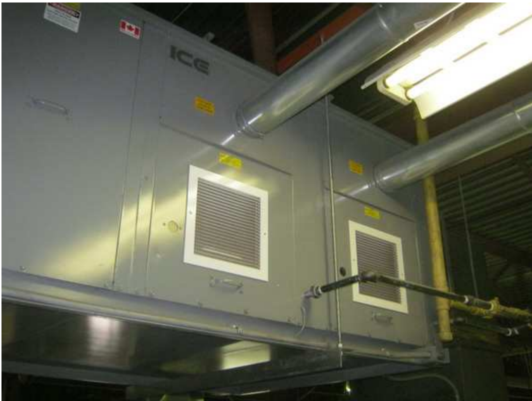
D304008-2 Newer ICG Packaged Heating Unit at Maintenance Shop
