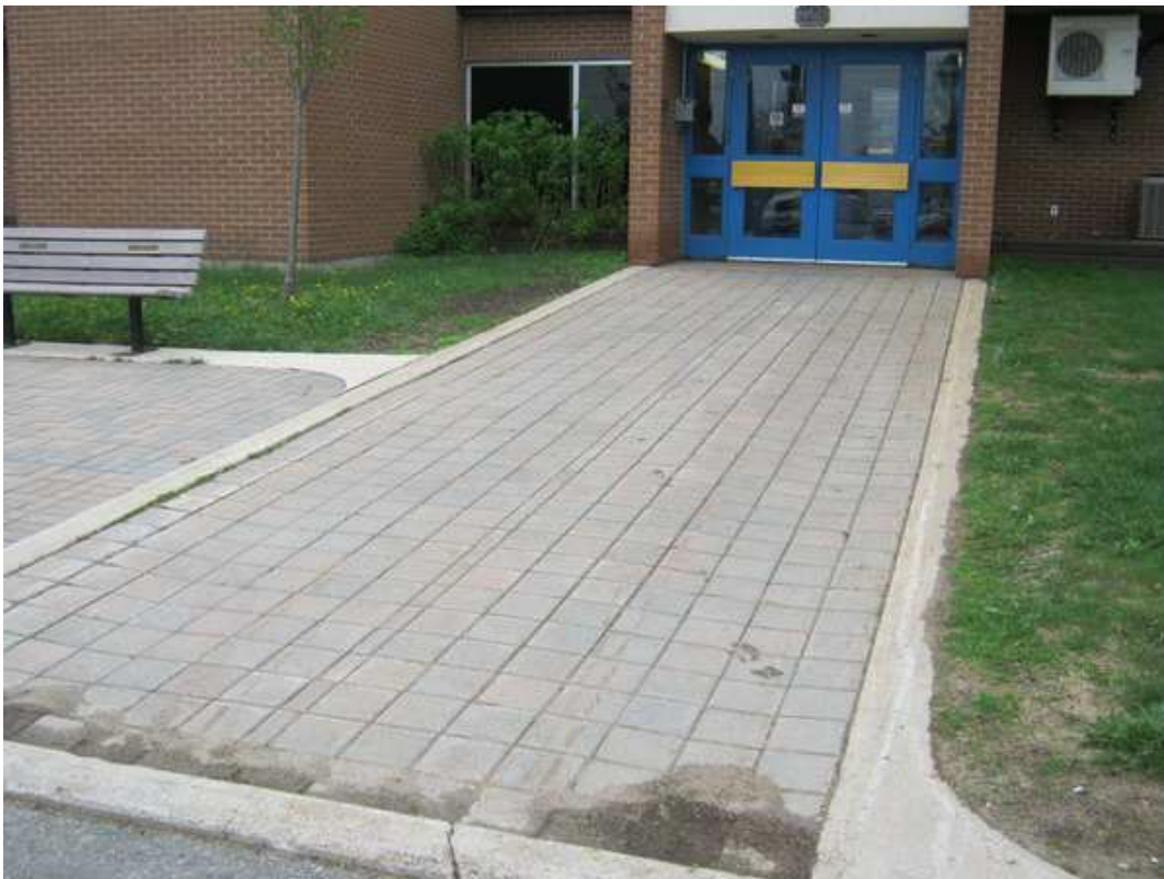
B203002a Note corrosion at base of entrance door
