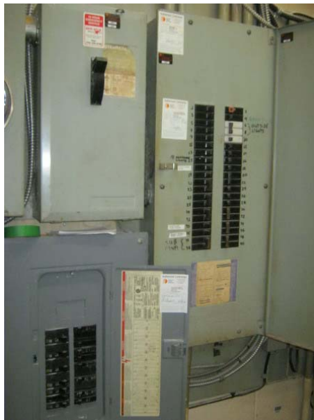
D501003 Electrical distribution equipment
