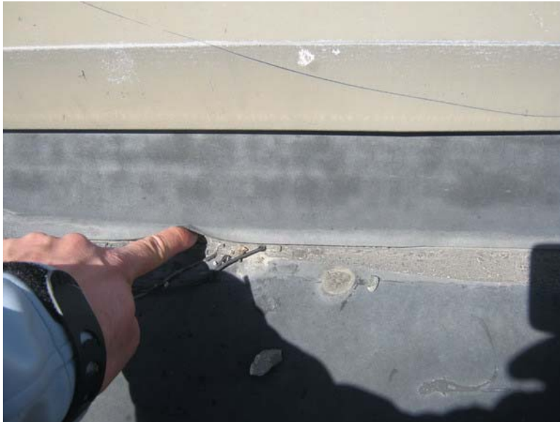
B3010a Debonding EPDM membrane at seams
