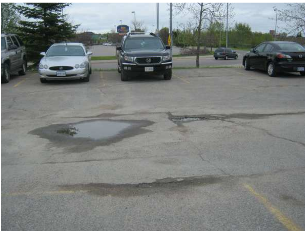
G202003a Partial view of staff parking, showing potholes and cracking asphalt
