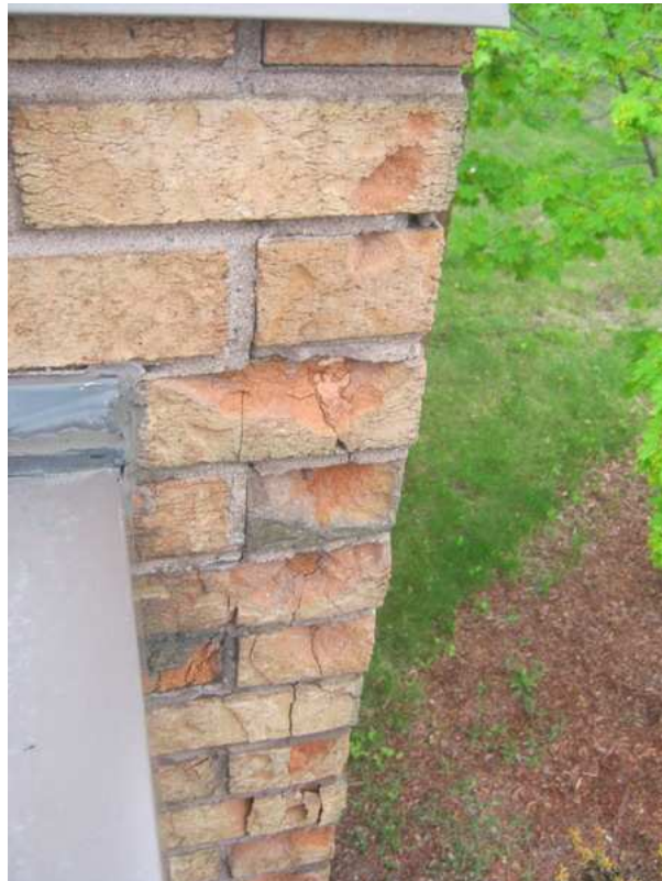
B2010a Deteriorating Brick Veneer at Entrance
