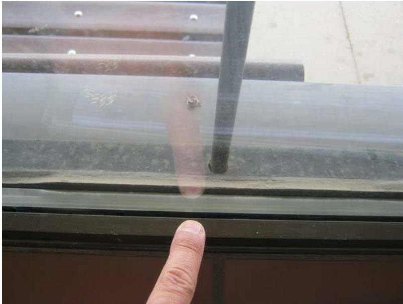
B2020b Fixed window missing interior glazing gasket
