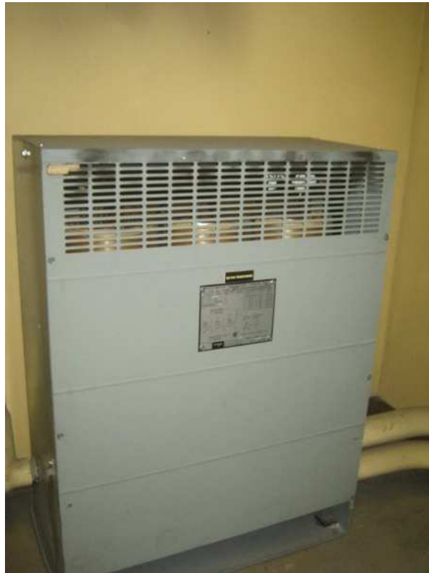
D501004a 150kVA Transformer in Electrical Room
