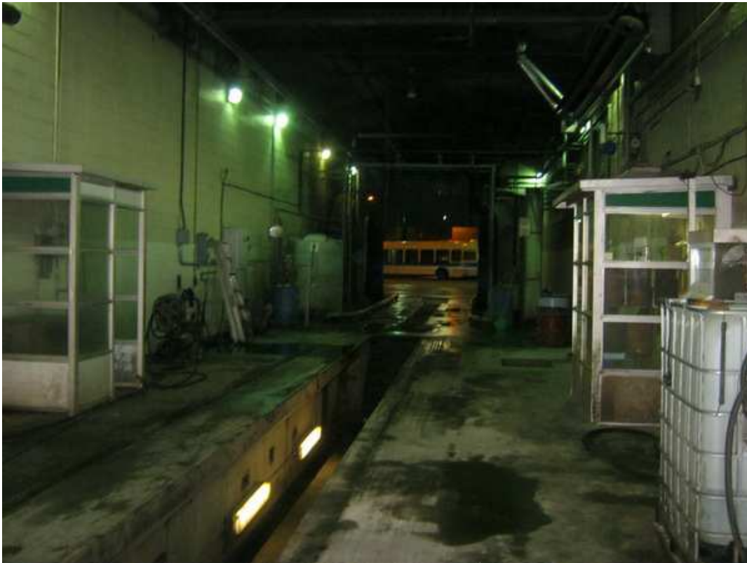
D509005 Wash Bay with buried Electrical Heating System
