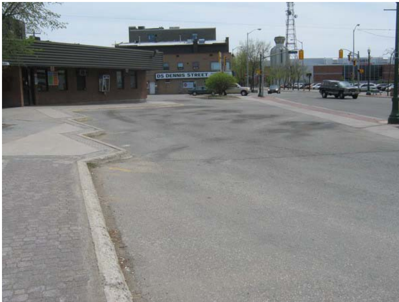
G202003 Asphalt at bus bays
