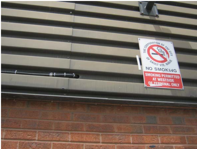
B201011 Penetration through metal cladding not sealed
