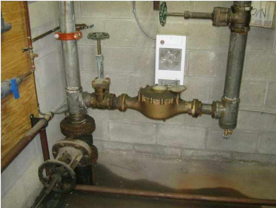
D202001 Incoming Water Service
