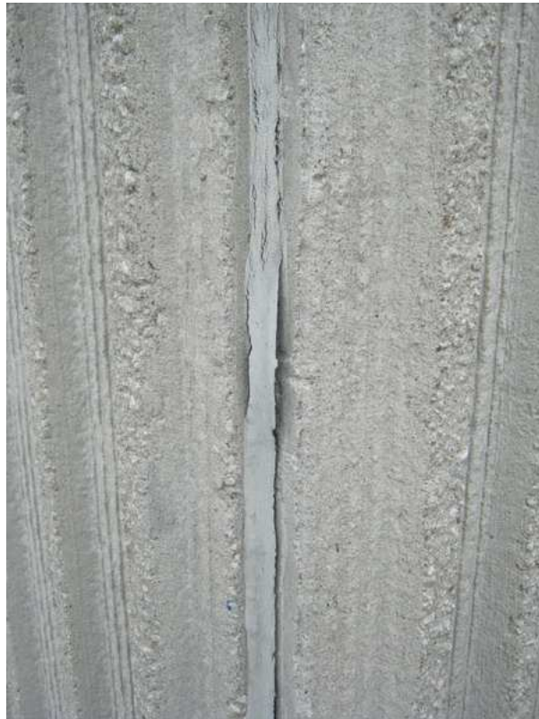
B201011 Deteriorated Sealants are Debonded and Crazed.
