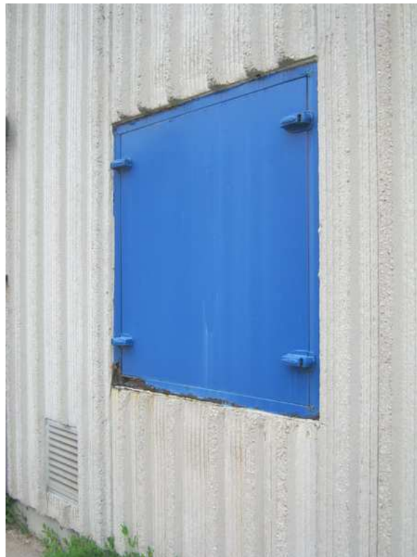
B203006 Blast Door from Paint Room
