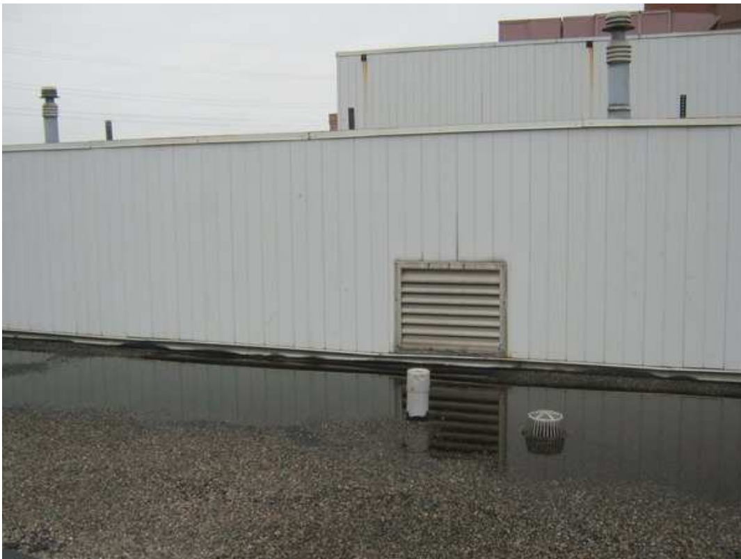
B3010b Ponding Water at Wall to Upper Roof
