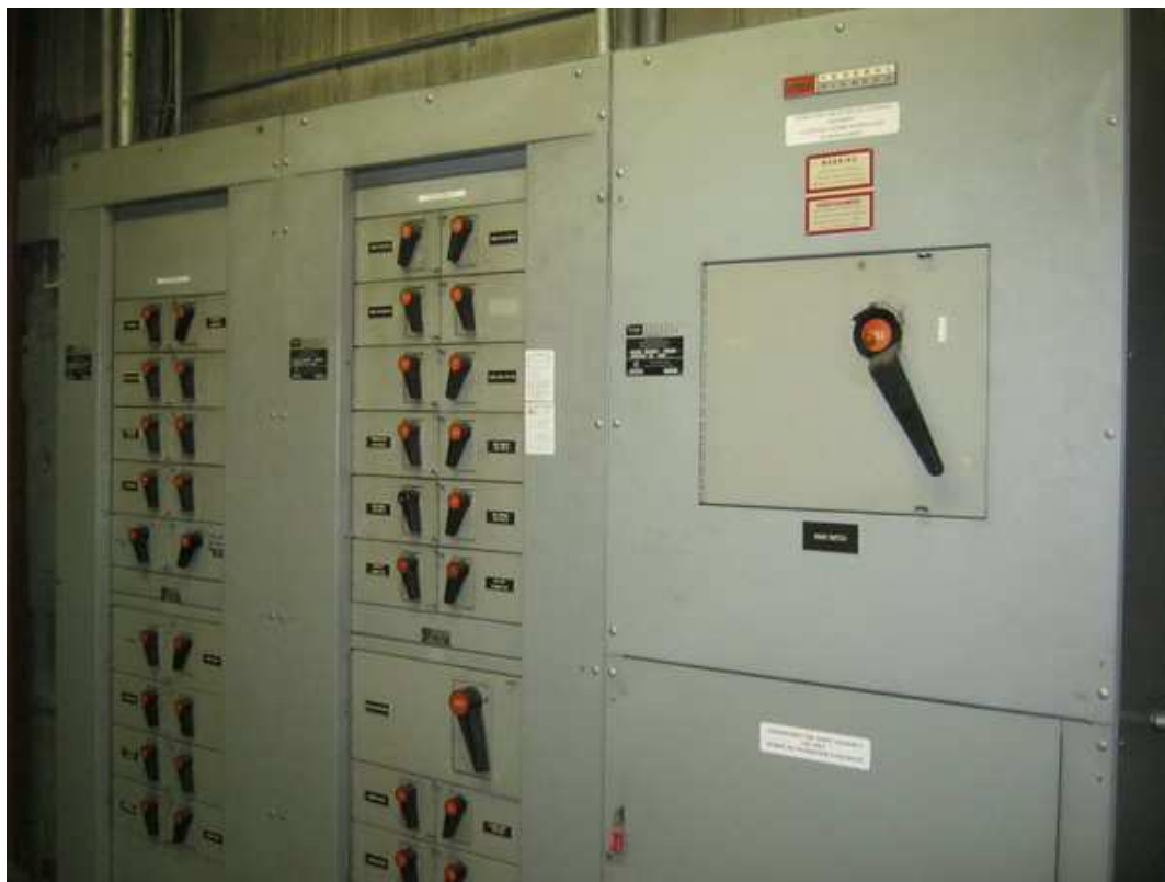
D501003 Main 600Volt Electrical Distribution Board
