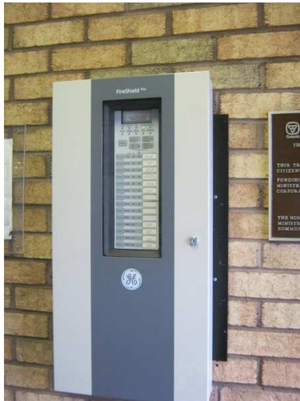
D503001 Overview of Fire Alarm Panel
