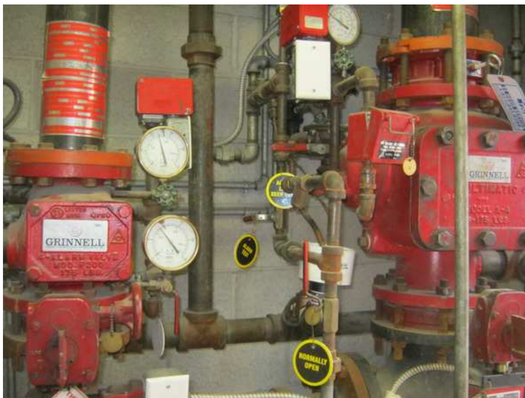
D401002 Overview of Sprinkler Distribution Equipment
