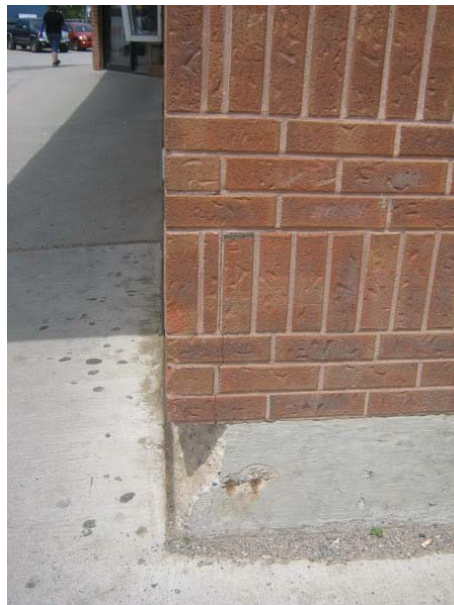
A10 Spall in Concrete Foundation
