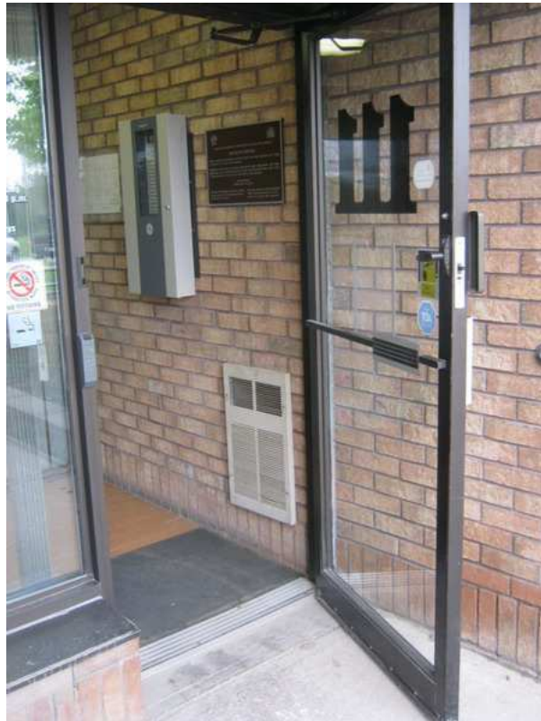
B203002b Powered Entrance Door does not open fully
