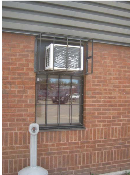
D303002 Window in drivers lounge with air conditioner
