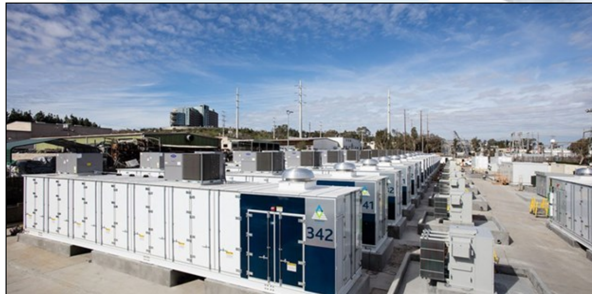
Example of a 30MW/120MWh system installed by Fluence in the San Diego area
