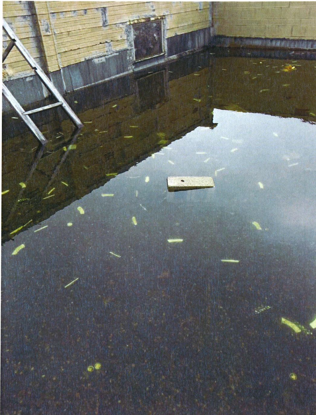
Photo No. 3 Roof Ponding. Approximately 50'x50' This area must be drained.
