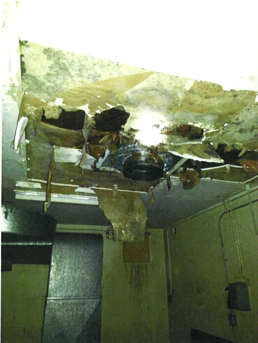
Photo No. 4 Example of ceiling finishes falling away from roof and ceiling structures
